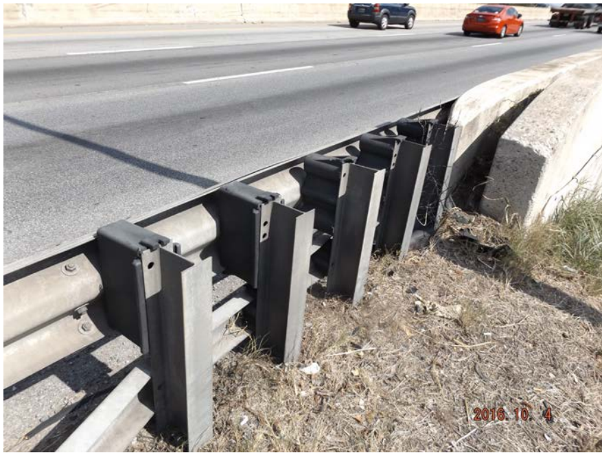
TRAFFIC SAFETY FEATURES - GUARD RAIL
